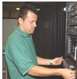
Larry Shepard , System Administrator, IS/IA Support, finishes racking another server for the ATC Active Directory test environment.
